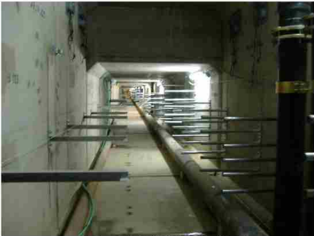
Gambar 2.10. Haifa Utility Tunnel, Israel
