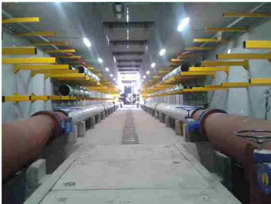
Gambar 2.12. Utility Tunnel Gandhinagar, India
